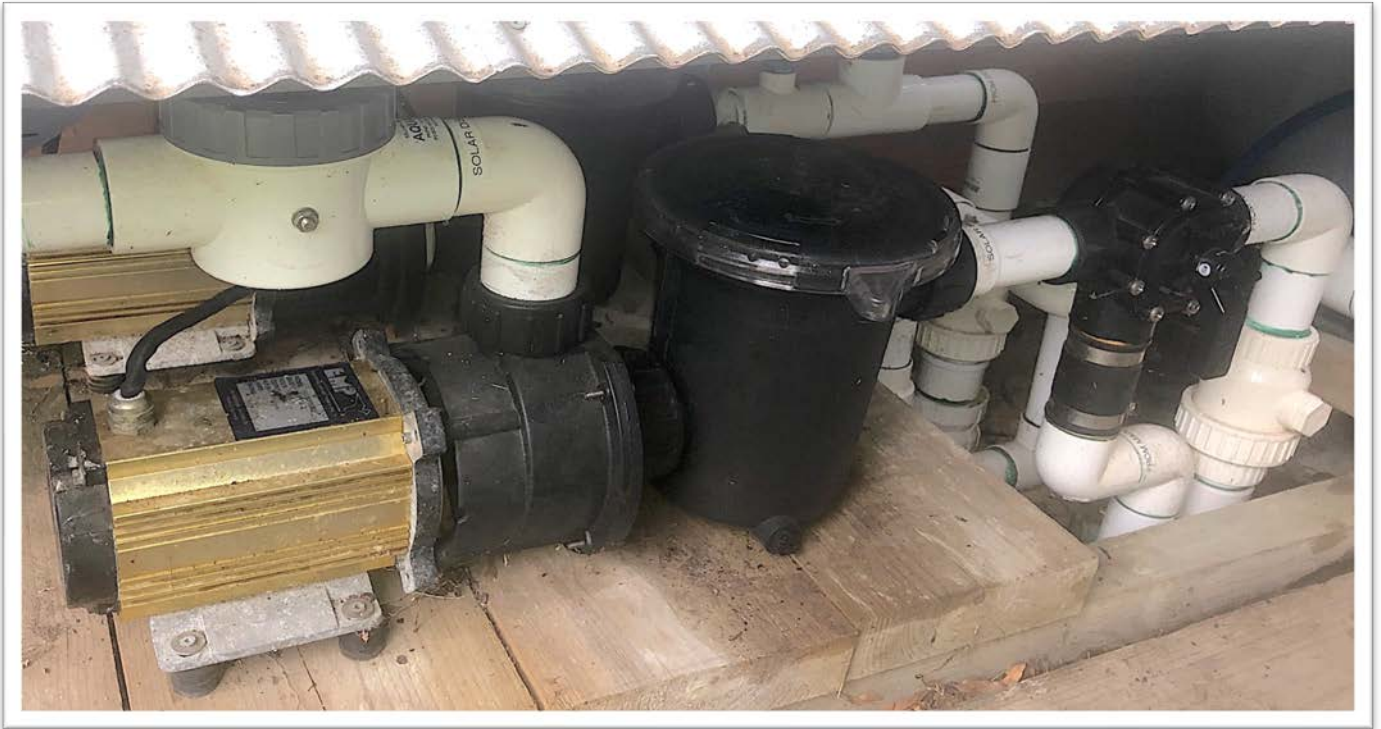
Pic.1: 500 Watt filtration / ionising pump on the company's pool. Normally set to 350 Watts max.
