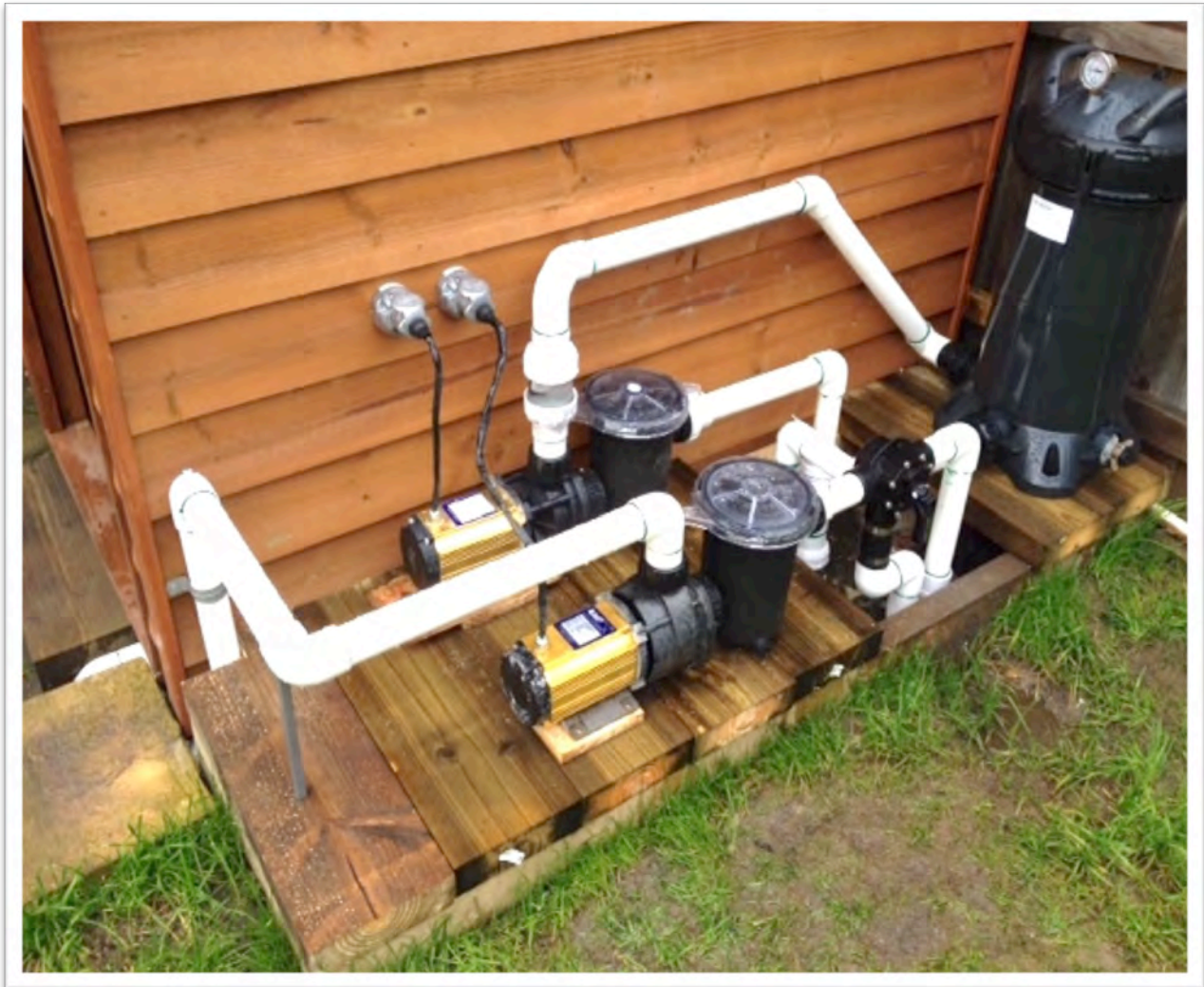
The two 48V DC (off grid) pumps on the company's 65,000 litre demo pool.
